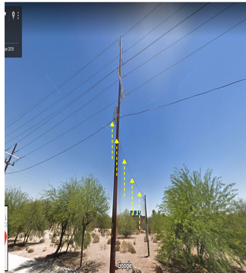
Figure: An overhead line going underground.
