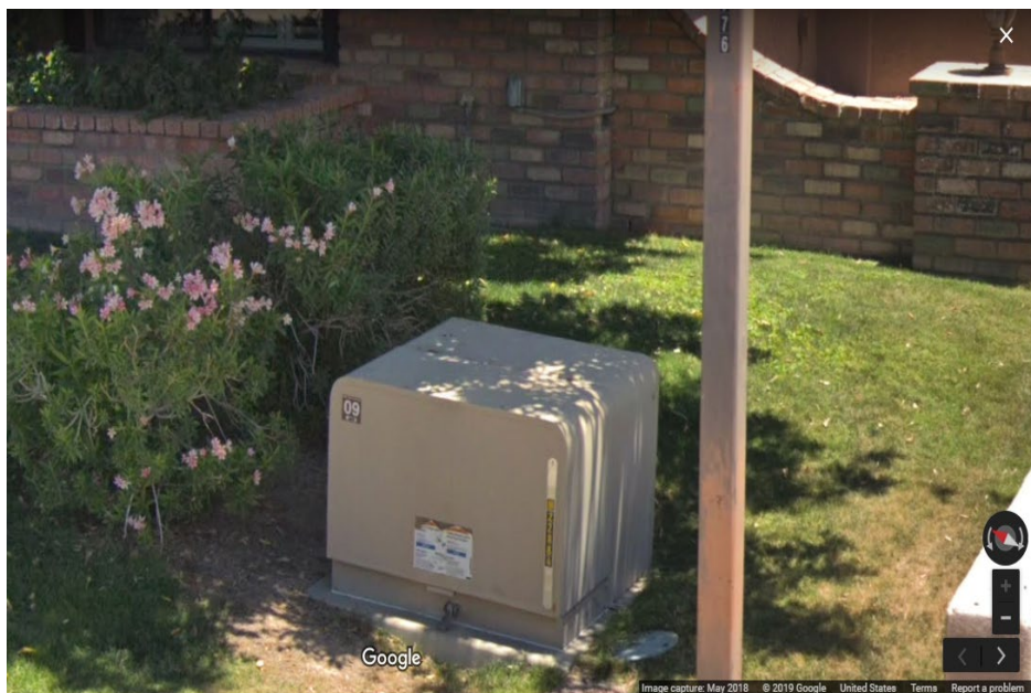
Figure: A pad mounted transformer for underground distribution.
